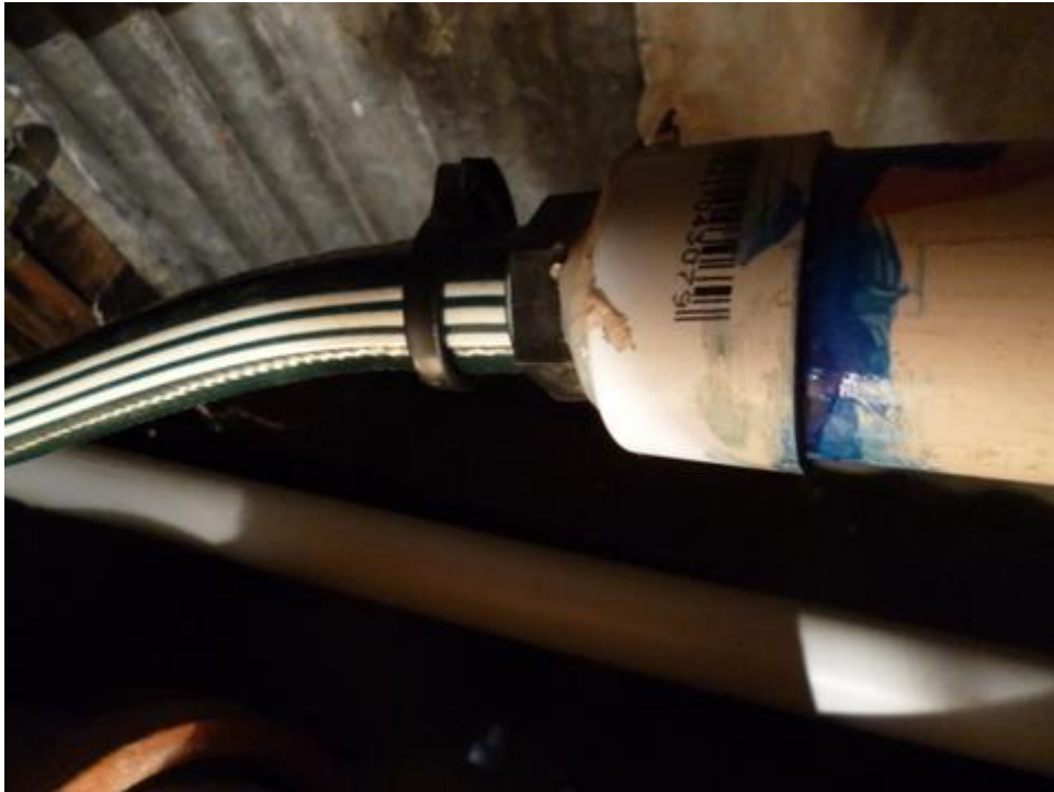
Line coming out the front of the valve, out through a ventilation gap in the bricks and into the banana circle
