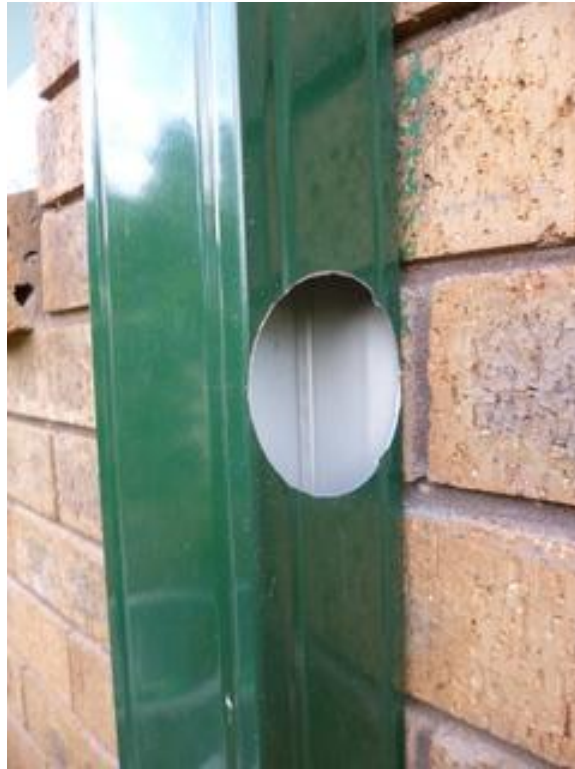
Holes cut in downpipe
