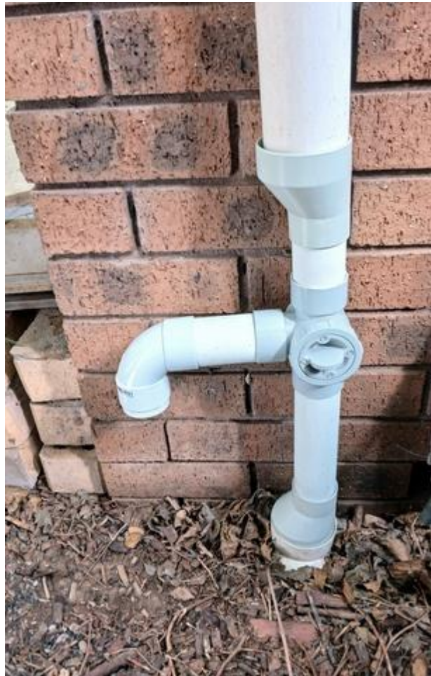
Valve setup in place
