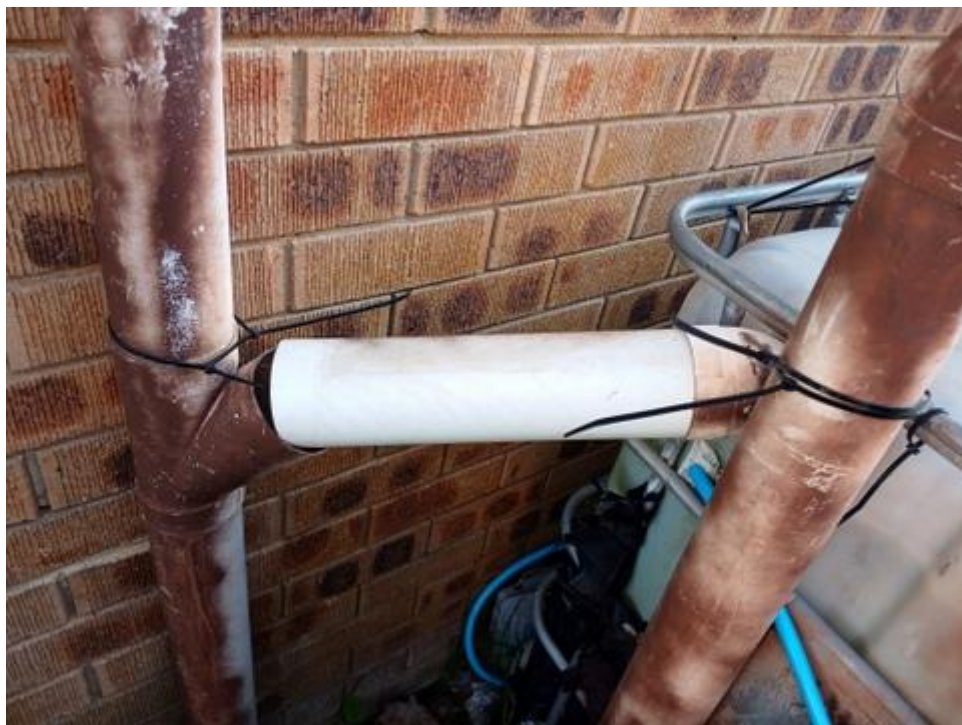
When full the IBC overflows via this pipe into a nearby downpipe
