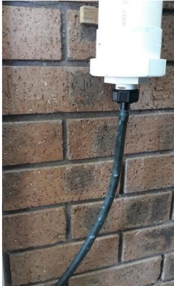
First flush drain, with timber bracket near the top of the pic
