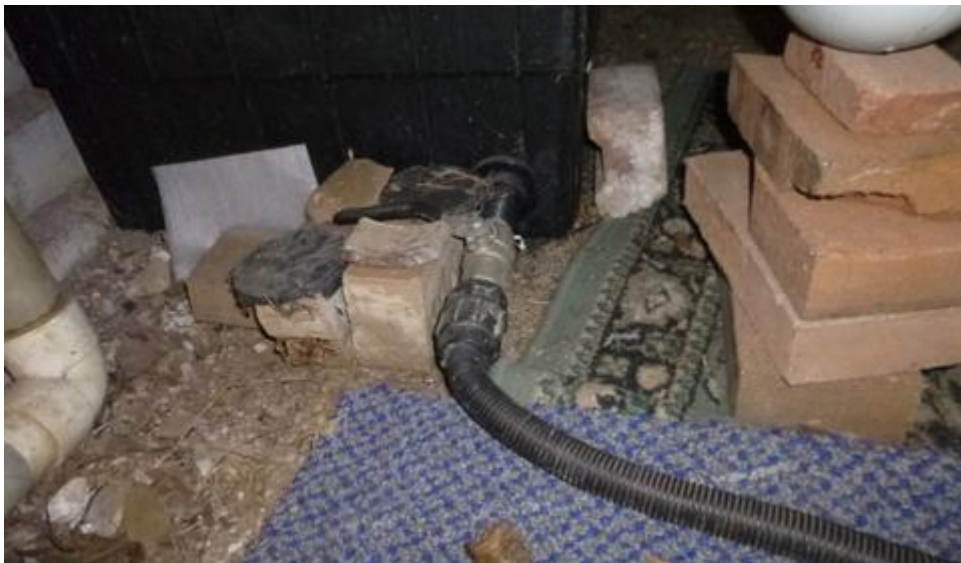
Pit drain to allow cleaning
