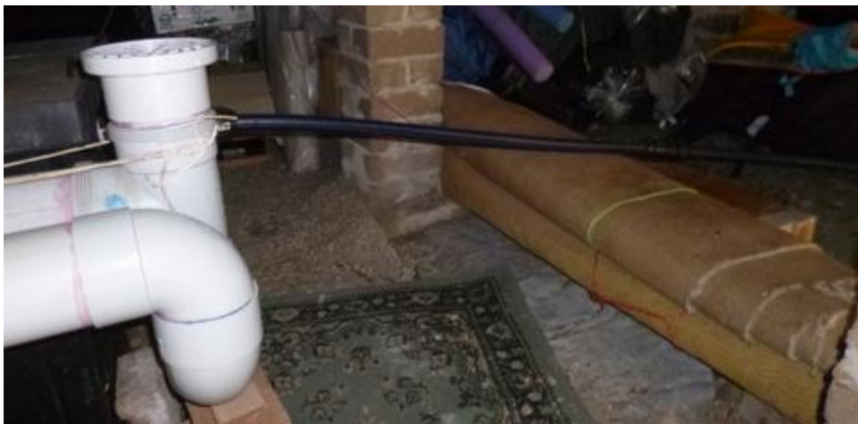
Output, through the pump, to the treatment area
