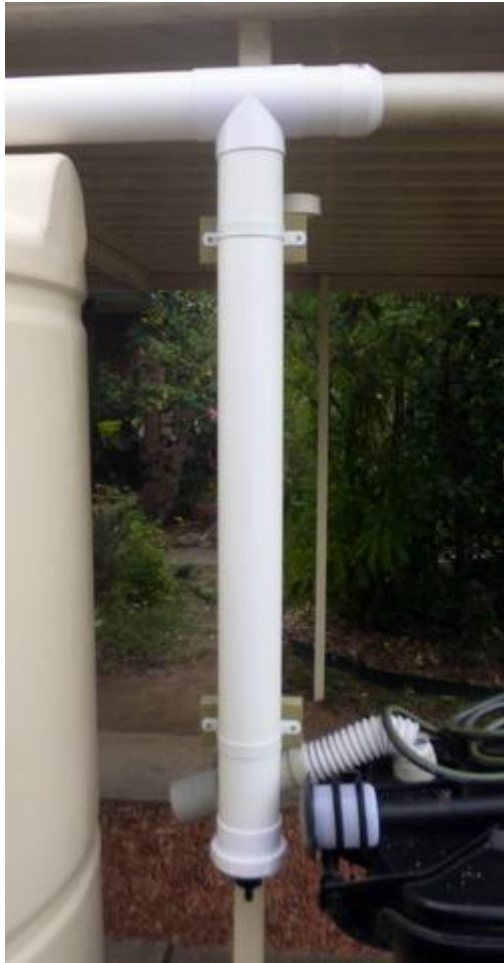
First flush diverter on one of our tanks
