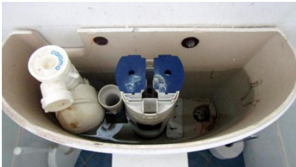
The view inside our cistern - white structure on the left is the inlet, open tube in the middle is the internal overflow and the cylinder on the right is the dual flush mechanism.
