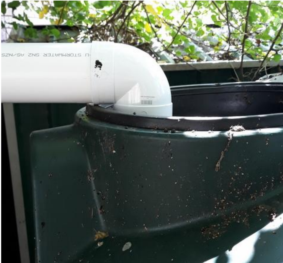
System outflow into the tank
