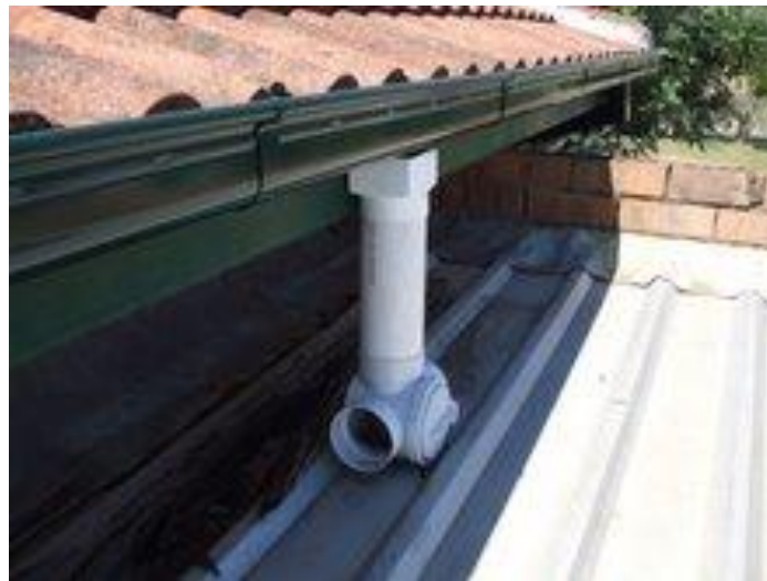
Extra downpipe to garage roof with valve
