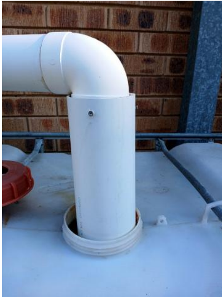
Rainwater gets directed into the top of the IBC
