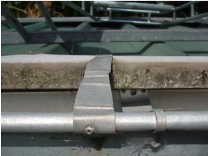
This shot shows a brace, pop riveted on the roof, curled around the gutter and pop riveted to the gutter
