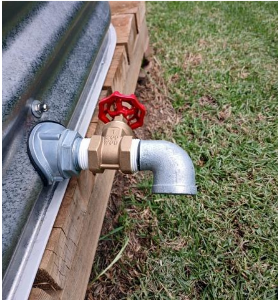
New outlet valve
