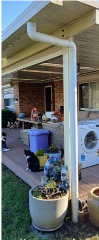
Downpipe from the gutter to the buried section of pipe
