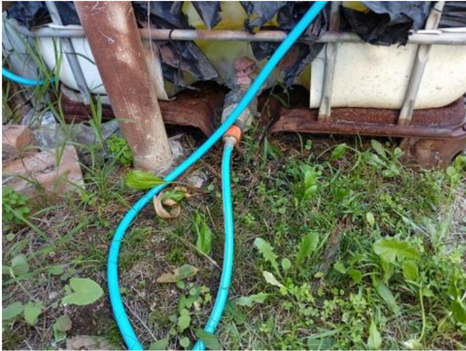
Tap and hose for accessing the water in the IBC
