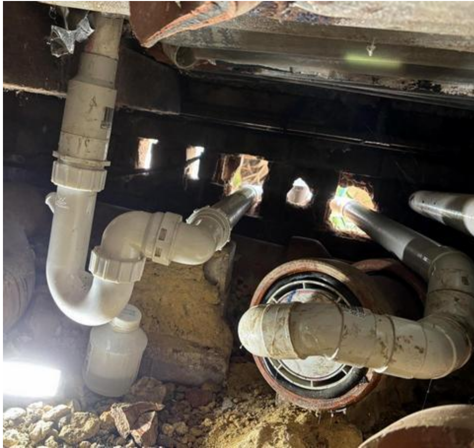
New system showing drain pipes now going out through the house back wall
