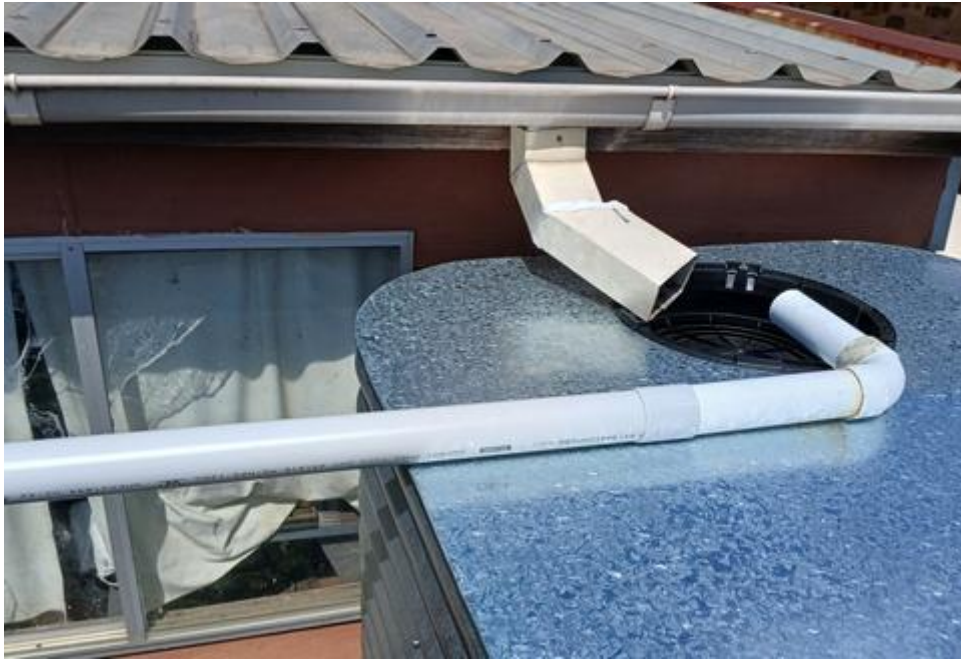
Overflow from the old tank goes into the new tank (hopefully)
