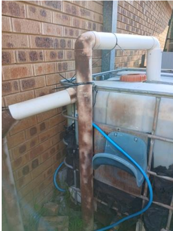
The pipes rise out of the ground next to the IBC to deliver the water into it
