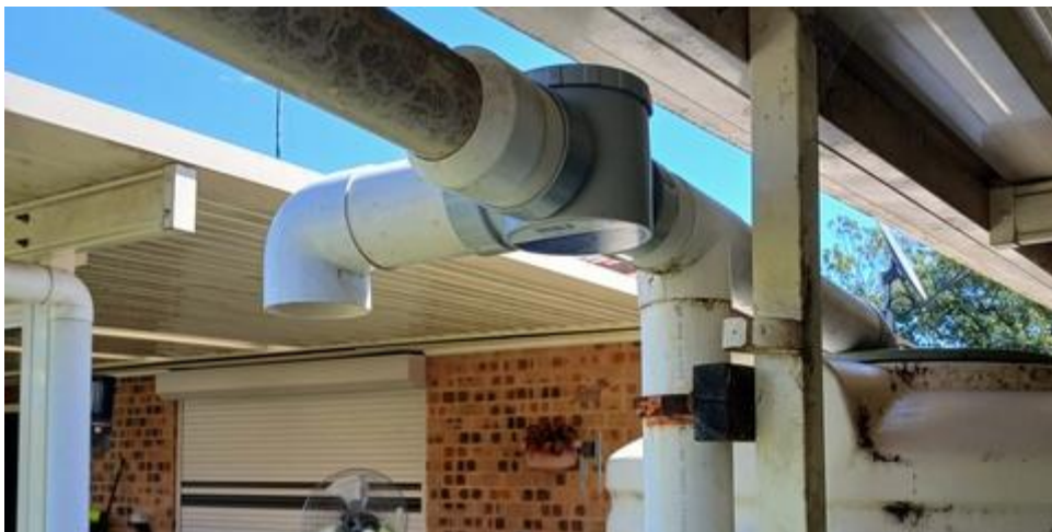
Leftward facing orientation of the valve outlet
