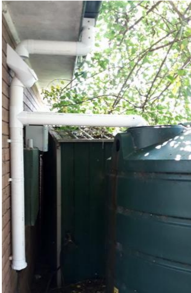
System in place and set up (tank overflow removed for clarity)
