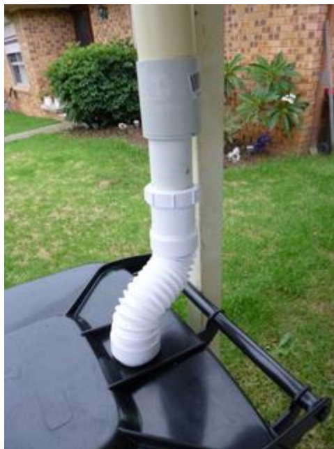
The Trap etc in place
