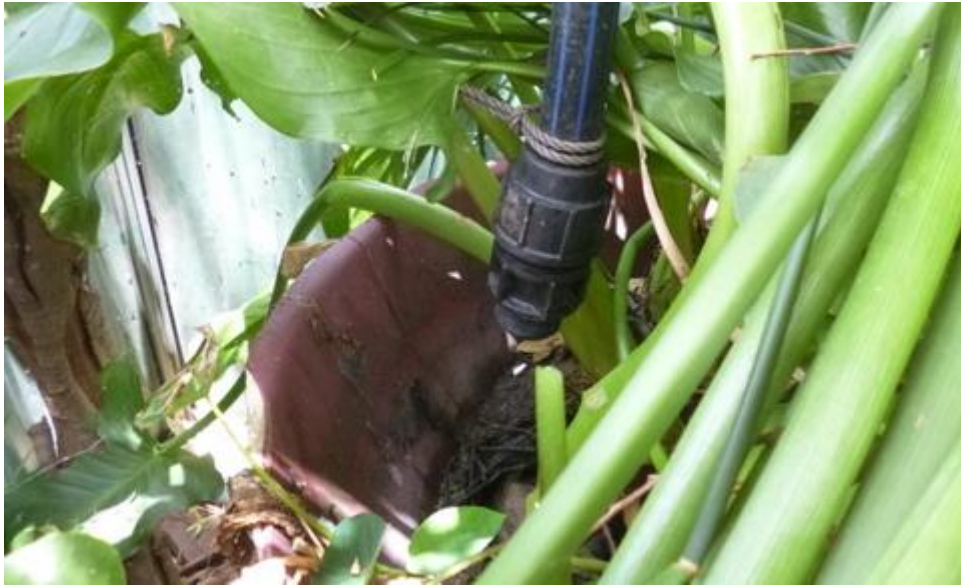
Hose discharging into the spa
